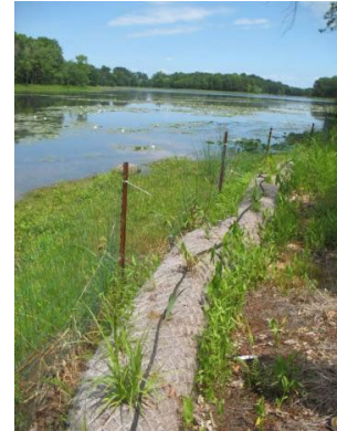
Site where biologists have been installed for additional stabilization and protection from waves
