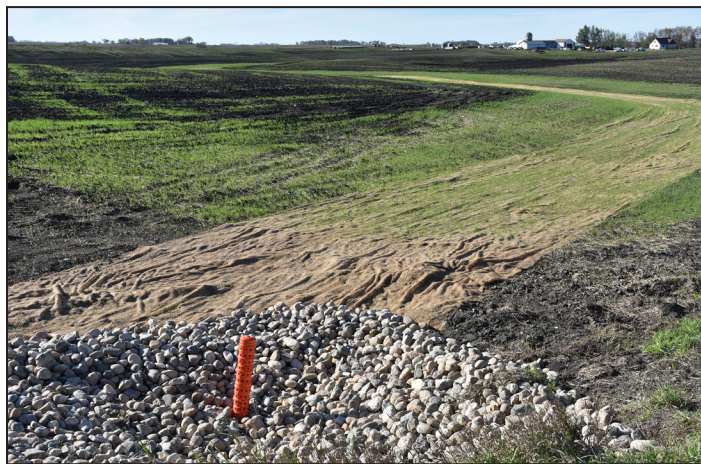
Erosion-control work affecting the South Branch Wild Rice River has water-quality benefits that extend to Lake Winnipeg.
