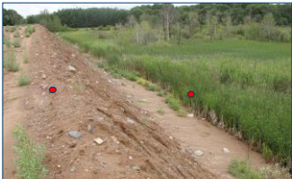
Recent, unauthorized fill that buried natural vegetation and native soils, and altered hydrology
