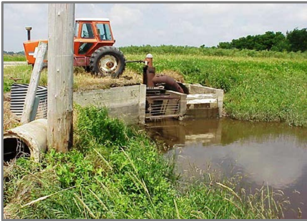
Figure 2. Drainage Pump Powered by Tractor's PTO
