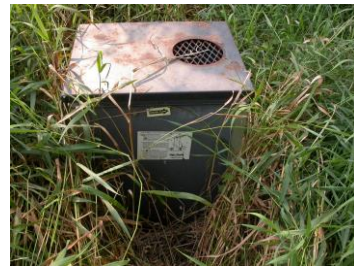
Water level control structure
