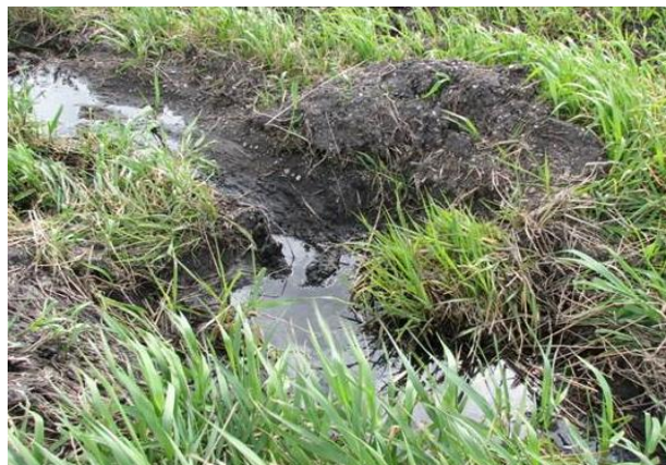
Figure 11. Eroded Channel above Settled Tile Block Trench
