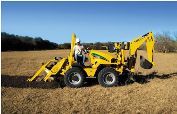
Figure 6. Supplemental Trenching to Aid in Destroying Subsurface Tile Within Sloped Wetland Settings
