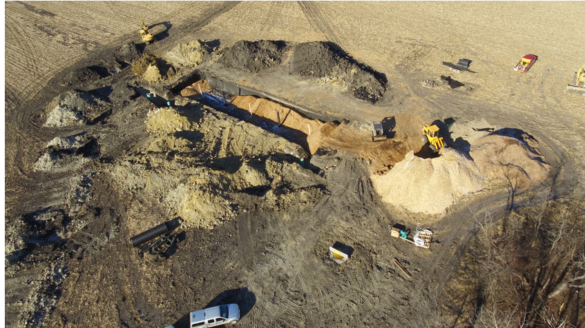
A drone image depicts a wood-chip bioreactor under construction in Fairbault County. Photo Credit: Fairbault County
