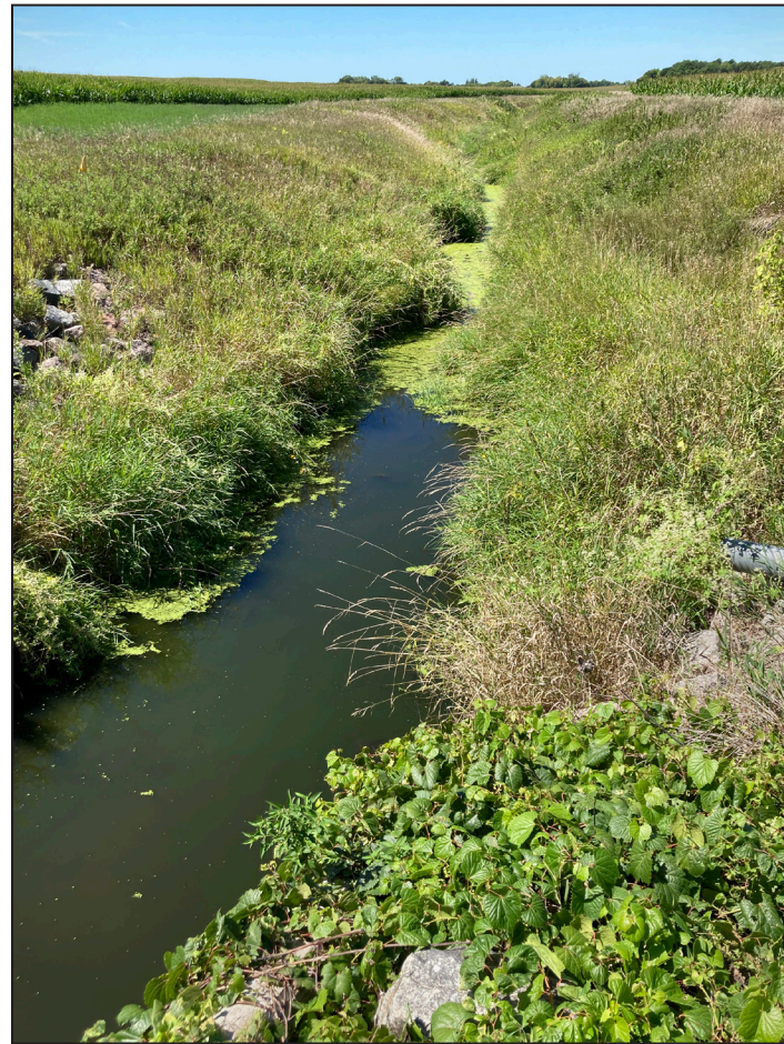
Judicial Ditch 111, formerly McLeod County Ditch 11, is seen Aug. 15, 2023, at a road crossing near Winsted. Photo Credit: Ann Wessel, BWSR
