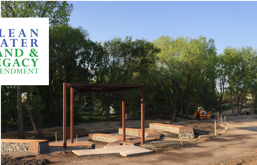
In Brooklyn Park, a trail connection and amphitheater-style overlook were constructed in conjunction with the Shingle Creek WMC stream restoration. Photo Credit: City of Brooklyn Park
