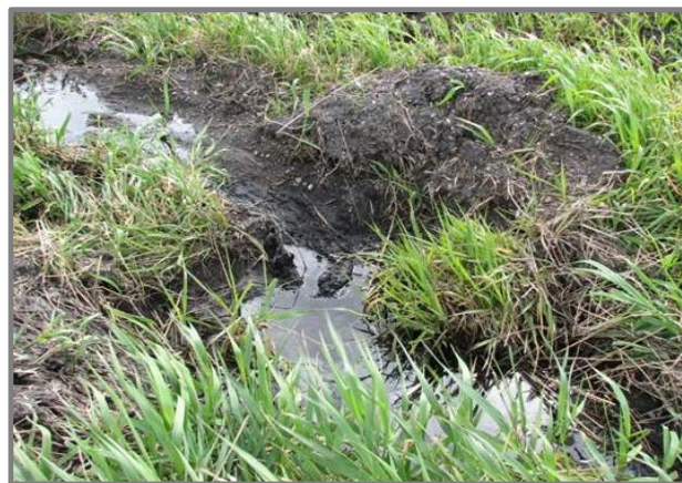
Figure 11. Eroded Channel above Settled Tile Block Trench
