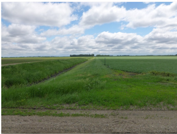
Pictured top to bottom, Ditch #9, #32 and #33 after side inlet and buffer strip installation.
